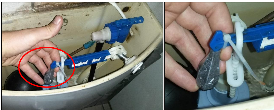
Figure 2: Fishing sinker attached to end of level arm inside toilet cistern to counter-balance siphon flush
